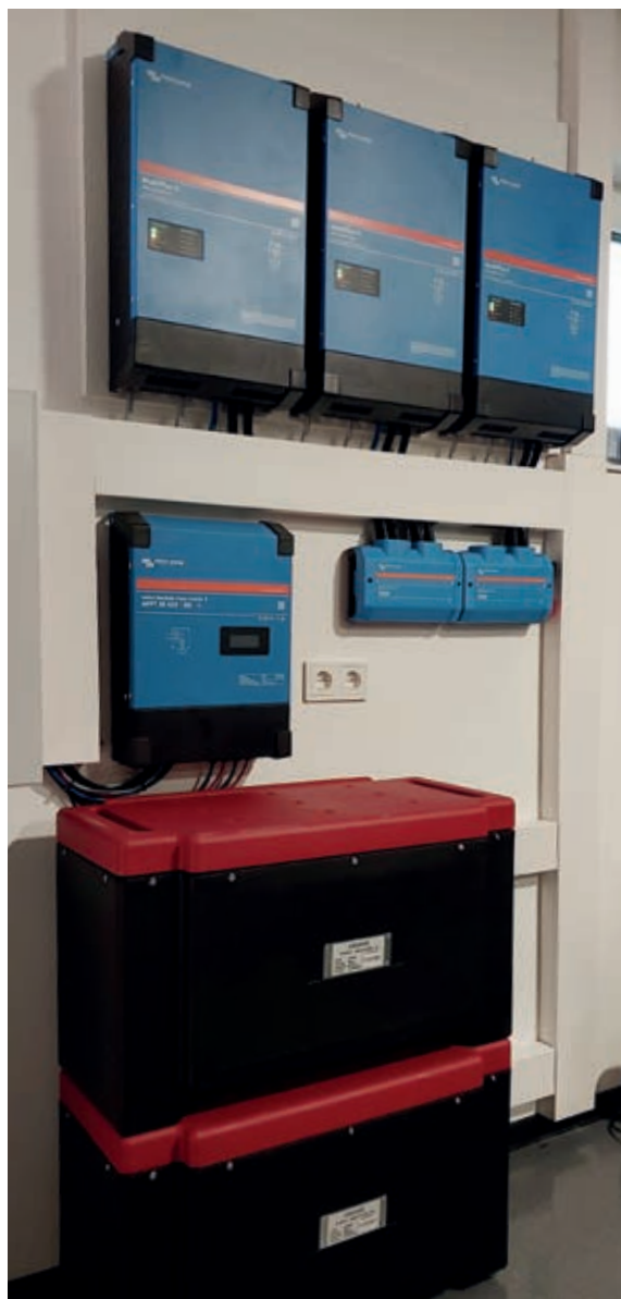
Victron & Cegasa ESS-System 3x3 kW + 27 kWh Speicher
